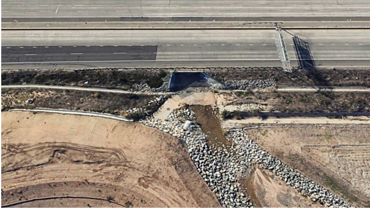
The north entrance to the tunnel extends under the 5 Freeway. Credit: Google Earth
